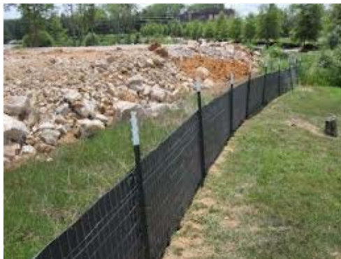
Figure 2: An example of a silt fence to control sediment and other debris
