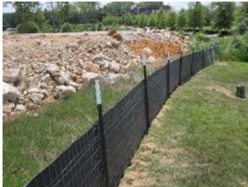
Figure 2: An example of a silt fence to control sediment and other debris
