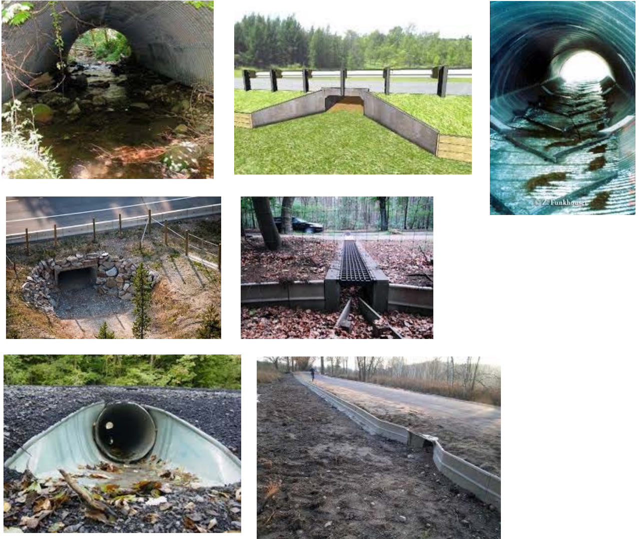
Figure 1: Examples of culverts to allow amphibians and small faunal species to cross roads
